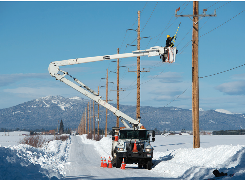
Idaho Power journeyman lineman operates a distribution switch on a 138-kV line in Valley County, Idaho. Photo courtesy Idaho Power.
